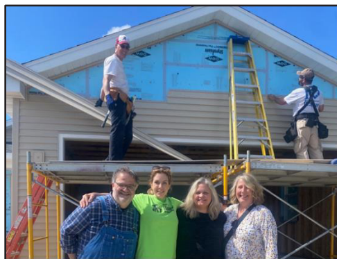
Pictured (left to right) at Habitat home #49: Jimmy Kaplan, Abby Newman, Jacinda Duffin and Laurie Flanagan. Paul Zeller and David Diller in background installing siding.
